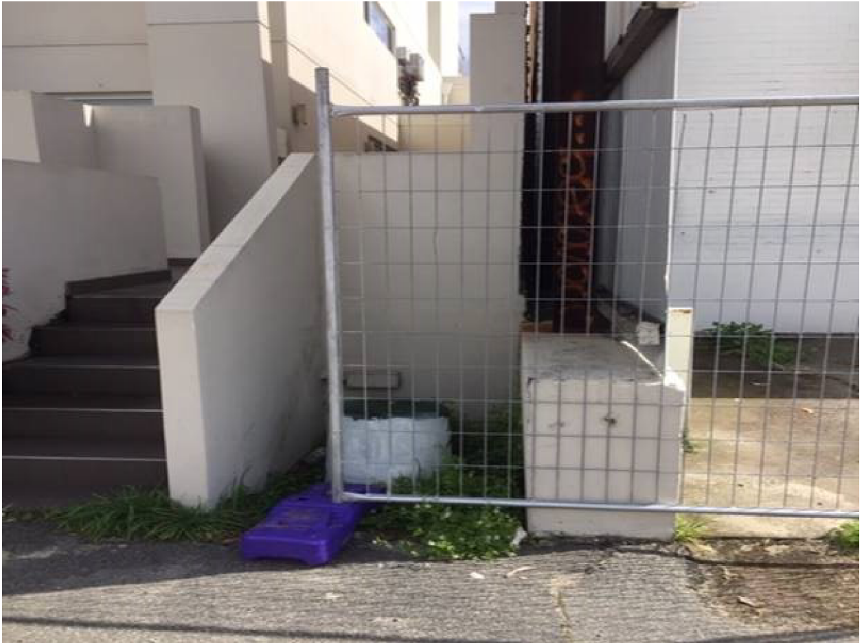
Vandals have put graffiti on the buildings.
