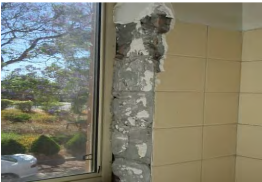
Figure 158 Missing Tiles Around the Window of the Kitchen
