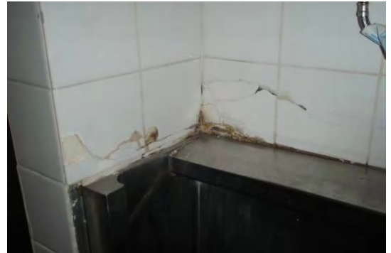
Figure 157 Broken Tiles and Corrosion in the Gentlemen's Toilet of the Bar
