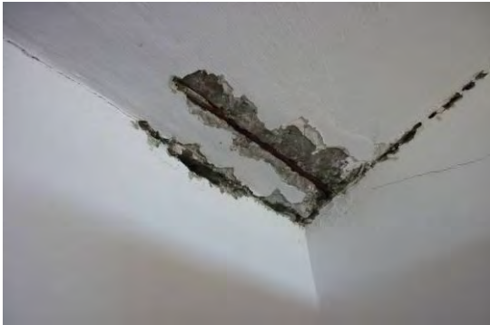
Figure 150 Concrete Cancer under Staircases in the Umpires Room
