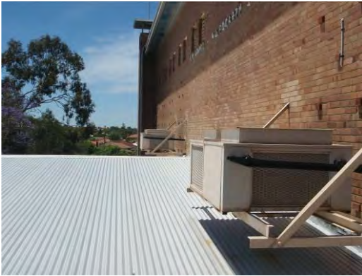
Figure 7 Redundant External Condensers
