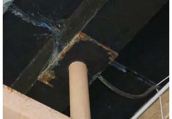
Figure 115 Steel Plate Rusted under Main Stand (West Side)
