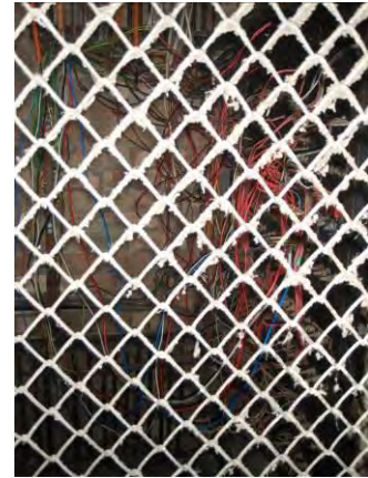
Figure 33 Function Room Electrical Switchboard Wiring
