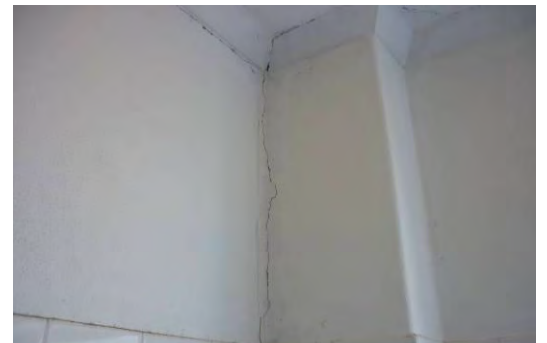
Figure 155 Crack in Wall and Ceiling in the Gentlemen's Toilet of the Bar
