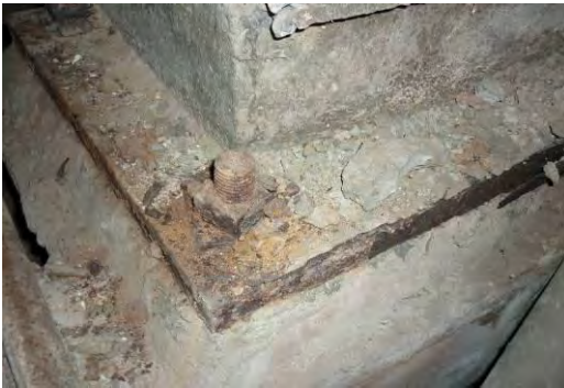
Figure 146 Bolts and Steel Plate Rusted at the Base of a Column in the Pumps Room
