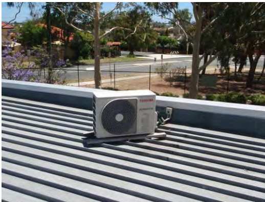
Figure 3 External Condenser Unit Not Securely Mounted
