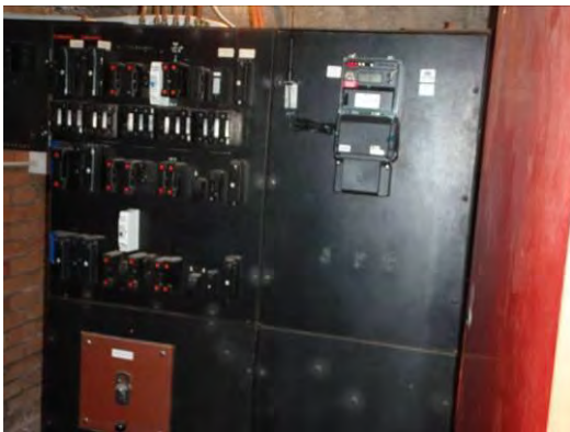
Figure 24 Building Main Switch Board (BMSB)
