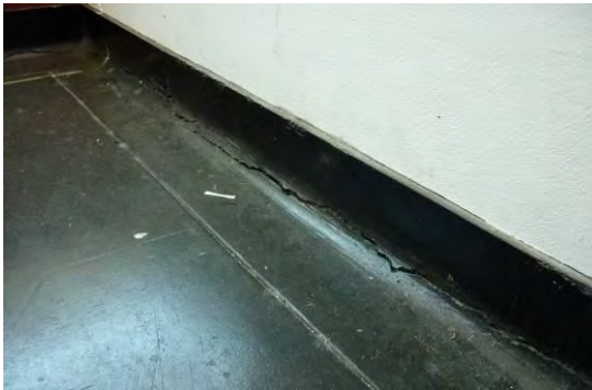
Figure 152 Crack between the Floor and Wall of the Umpires Room
