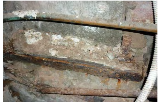
Figure 145 Bolts and Steel Plate Rusted at the Base of a Column in the Pumps Room
