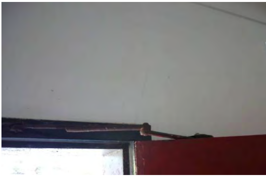
Figure 134 Crack Above Door Frame in the Ladies Toilet of the Ground Floor
