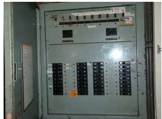
Figure 35 Function Room Electrical Switchboard
