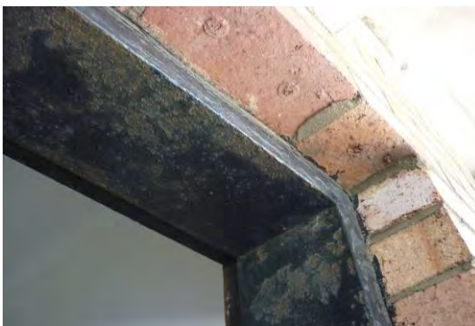
Figure 136 External Steel Door Frame Rusted in the Ladies Toilet of the Ground Floor
