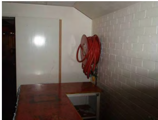
Figure 43 Fire Hose Reel – Back of Function Room
