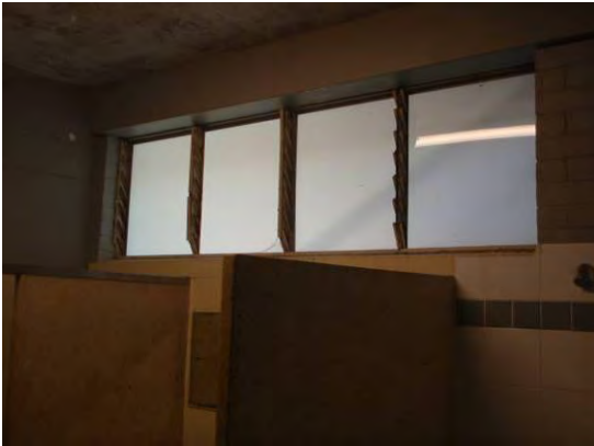
Figure 81 Visitors Shower Area
