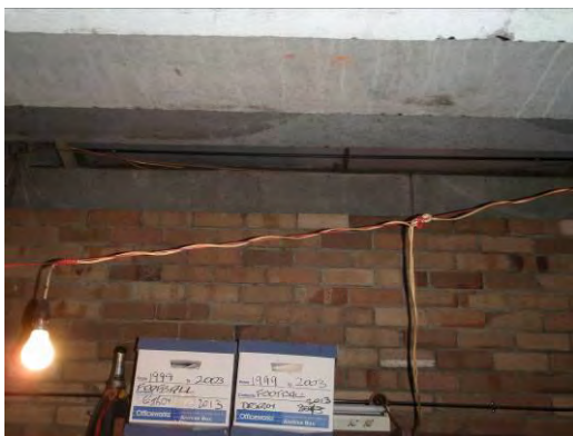
Figure 38 Lighting Cabling Function Room Store
