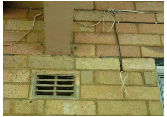
Figure 117 Crack in the Brickwork under Main Stand (East Side)
