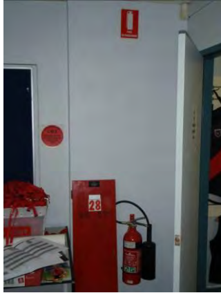
Figure 41a&b Office Fire Extinguisher
