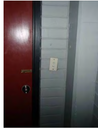
Figure 23 Light Switch Loose and Askew
