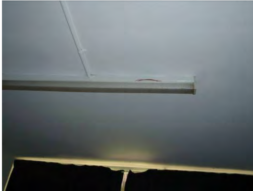
Figure 16 Cable 'Trapped' on Lighting Fitting Cover
