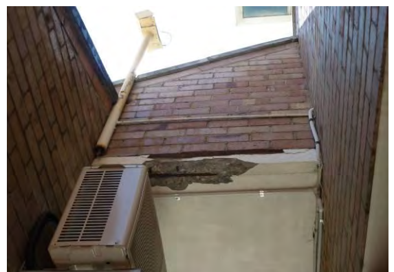
Figure 107 Concrete Cancer Outside the Changing Room
