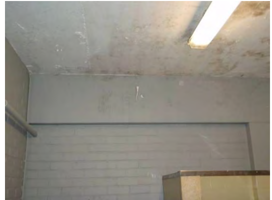
Figure 82 Visitors Shower Area Ceiling Damage
