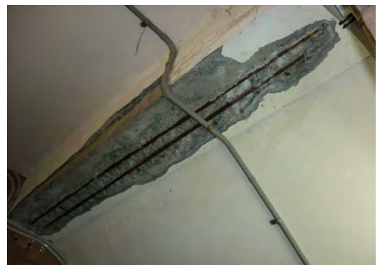
Figure 131 Concrete Cancer under the Staircase
