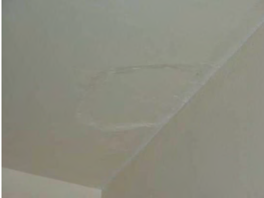
Figure 102 Water Leaking in the Massage Room
