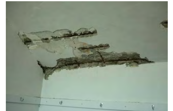
Figure 149 Concrete Cancer under Staircases in the Umpires Room
