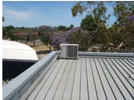
Figure 4 External Condenser Unit Not Securely Mounted
