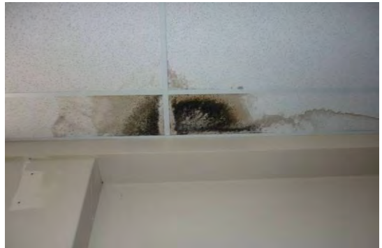
Figure 153 Water Leaking Stain in the Ceiling of the Function Room
