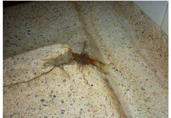
Figure 139 Cracks in the Floor of the Showers
