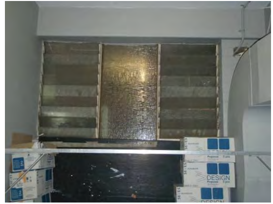
Figure 76 Visitors Changing Room Windows/Louvres
