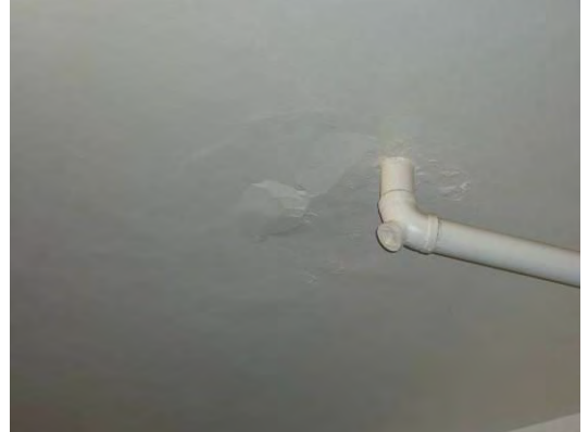
Figure 103 Water Leaking above Door Frame
