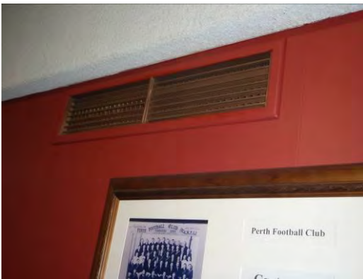
Figure 9 Redundant Air Supply Grille in Office
