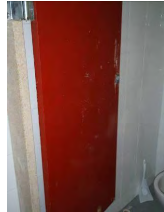
Figure 58 Perth Football Club Toilet Door
