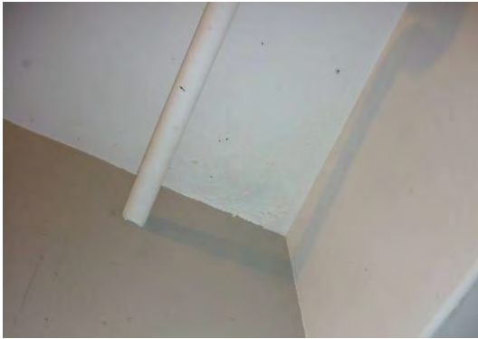
Figure 138 Water Leaking Stains in the Ceiling of the Toilet
