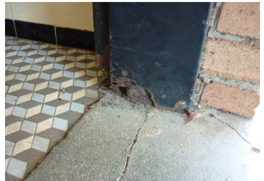
Figure 135 Crack in the Step and Steel Frame Rusted outside the Ladies Toilet of the Ground Floor
