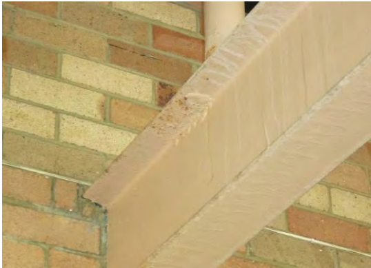
Figure 120 Universal Beam Rusted under Main Stand (East Side)
