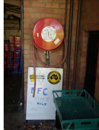
Figure 42 Fire Hose Reel – Ground Floor External
