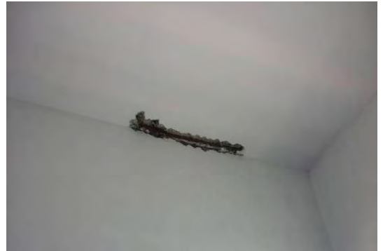
Figure 151 Concrete Cancer under Staircases in the Umpires Room
