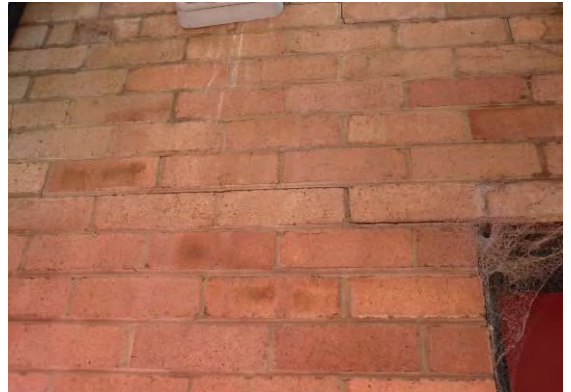
Figure 109 Crack above the External Door of the Equipment Room
