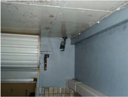
Figure 22 Faulty/Redundant Light Fitting
