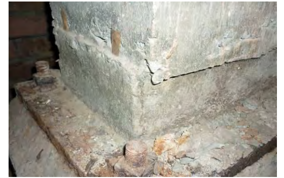
Figure 147 Spalling of Concrete at the Base of a Column in the Pumps Room
