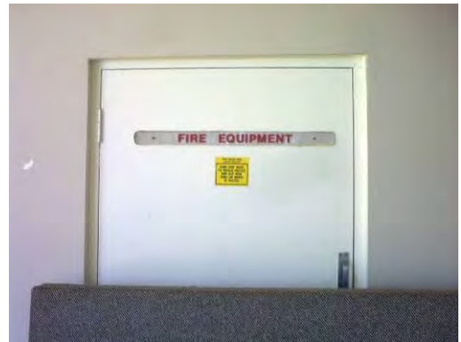
Figure 44 Fire Hose Reel – Function Room
