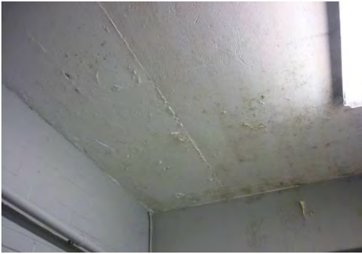
Figure 144 Water Leaking Stains in the Showers under the Bar
