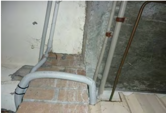
Figure 132 Crack Between Slab and Column under the Staircase
