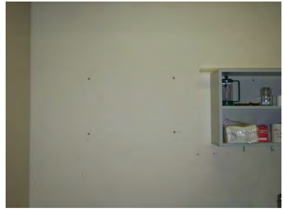
Figure 66 Office Area Old Screw Holes
