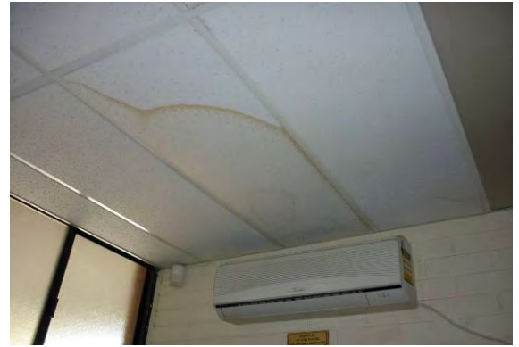
Figure 127 Water Leaking Stain in the Coaches Room
