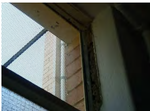
Figure 124 Poor Finish Around the Windows of the Toilet
