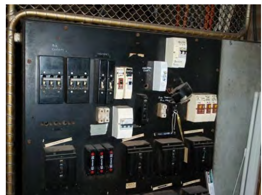
Figure 27 Function Room Electrical Switchboard 1
