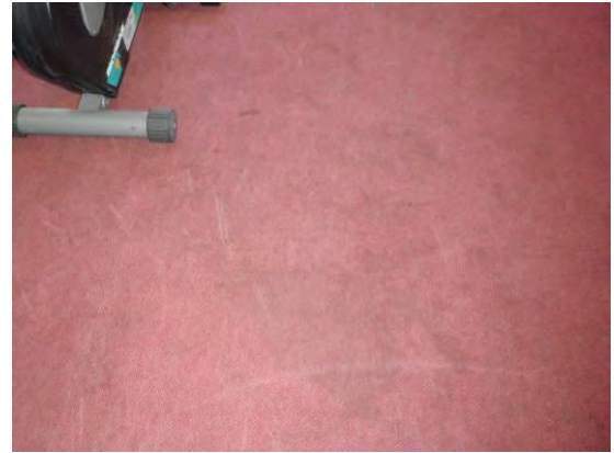
Figure 88 Office Area Stained Carpet
