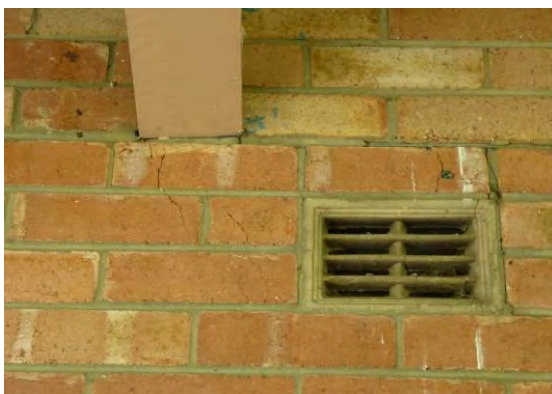
Figure 118 Crack in the Brickwork under Main Stand (East Side)
