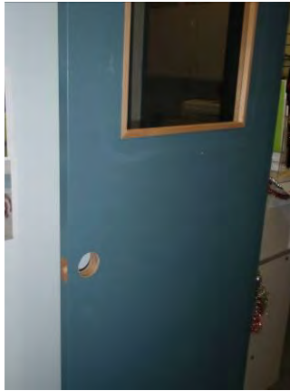
Figure 93 Office Door Missing Door Handle
