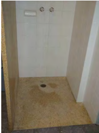
Figure 83 Visitors Shower Area Shower Cubicle
