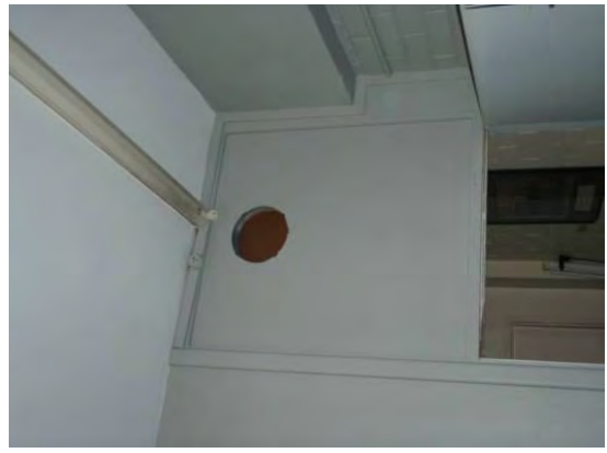
Figure 78 Visitors Changing Rooms Hole in Window Panel
