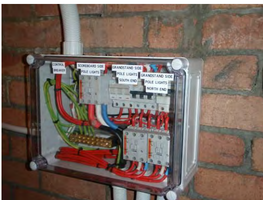
Figure 26 Grandstand Side Pole Lights Power Supply
