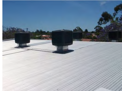
Figure 2 Evaporative Air Conditioning Units
