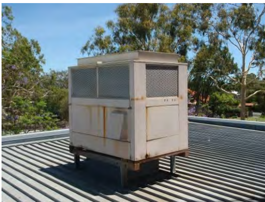
Figure 5 Redundant Evaporative (External) Air Handling Unit
