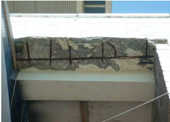
Figure 108 Concrete Cancer Outside the Changing Room
