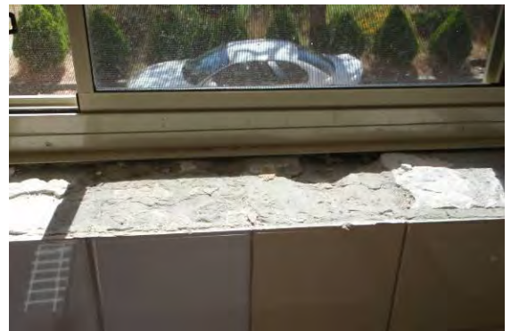
Figure 159 Missing Tiles Around the Window of the Kitchen
