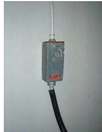
Figure 31 Visitors Changing Room Domestic Hot Water Isolator
