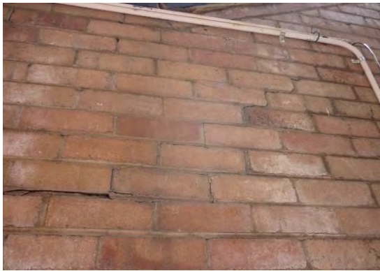
Figure 110 Crack above the External Door of the Equipment Room
