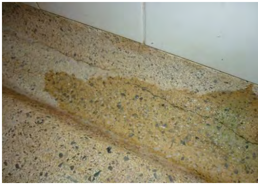
Figure 140 Cracks in the Floor of the Shower
