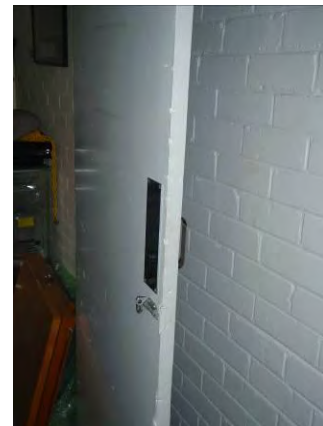
Figure 86 Visitors Area Damaged Door
