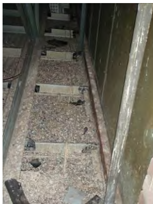
Figure 47 Grand Stand Roof Bird Droppings
