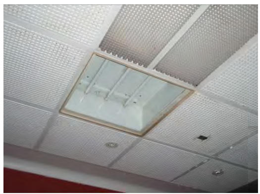
Figure 21 Function Room Diffuser Missing
