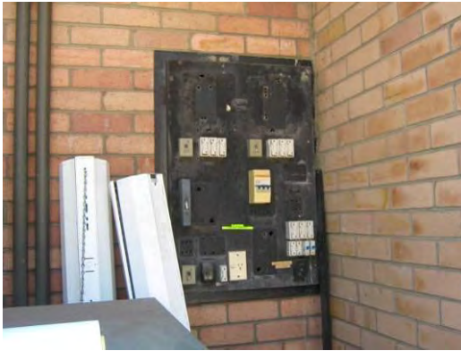
Figure 36 External Distribution Board (Possibly Redundant?)
