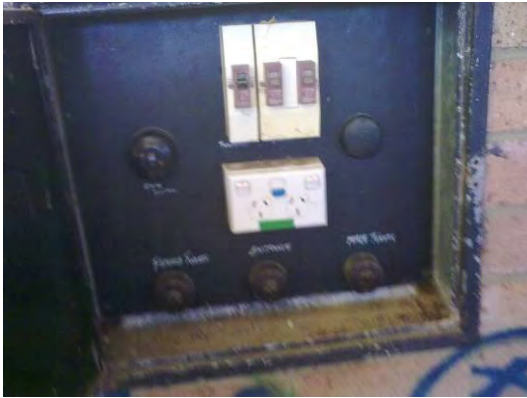
Figure 32 Function Room Electrical Switchboard
