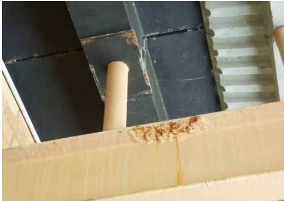
Figure 116 Universal Beam Rusted under Main Stand (West Side)
