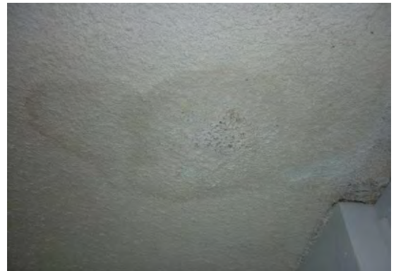
Figure 129 Water Leaking Stain in the Ceiling of the Administration Office
