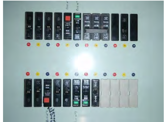
Figure 29 Function Room Electrical Switchboard
