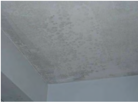
Figure 122 Water Leaking Stains in the Toilet of the President Lounge
