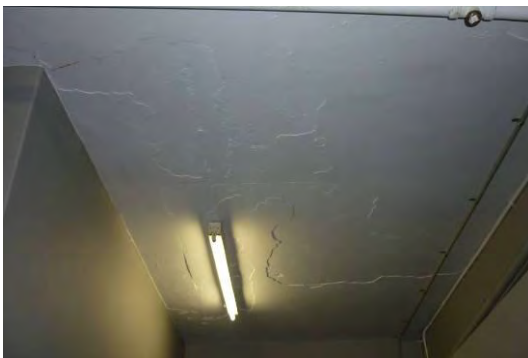
Figure 142 Previous Repair Works in the Ceiling
