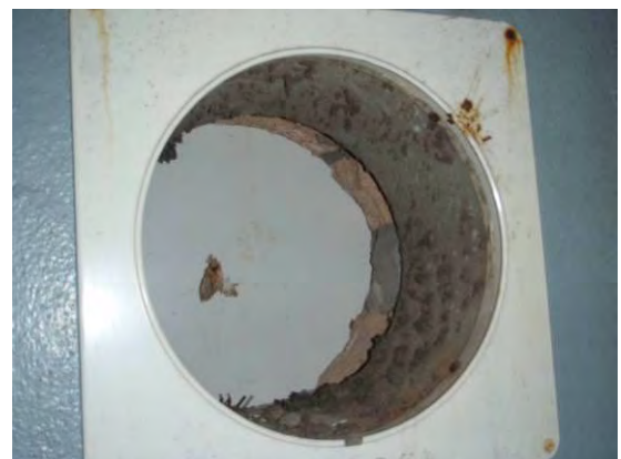
Figure 56 Perth Football Club 'Ice' Room Hole in Wall
