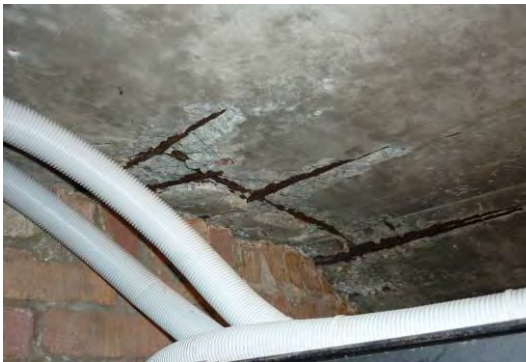
Figure 148 Concrete Cancer under the Stair Cases in the Switchboard Room
