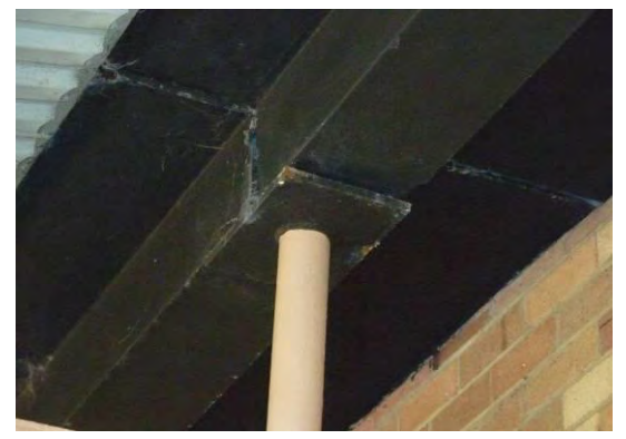
Figure 119 Steel Plate Rusted under Main Stand (East Side)
