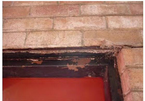
Figure 111 Equipment Room Door Frame Rusted
