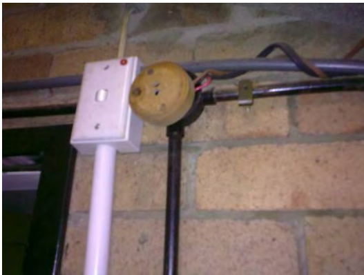
Figure 30 Function Room Store Electrical Connection
