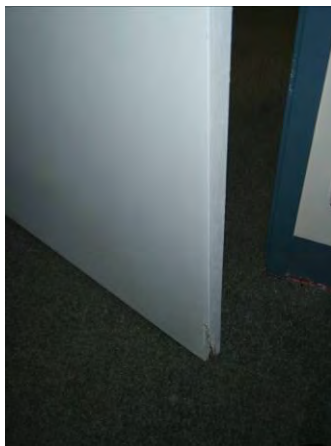
Figure 91 Office Area Damaged Door
