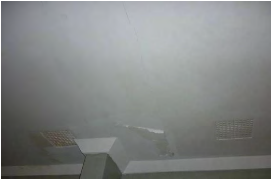
Figure 156 Crack and Water Leaking Stain in the Gentlemen's Toilet of the Bar
