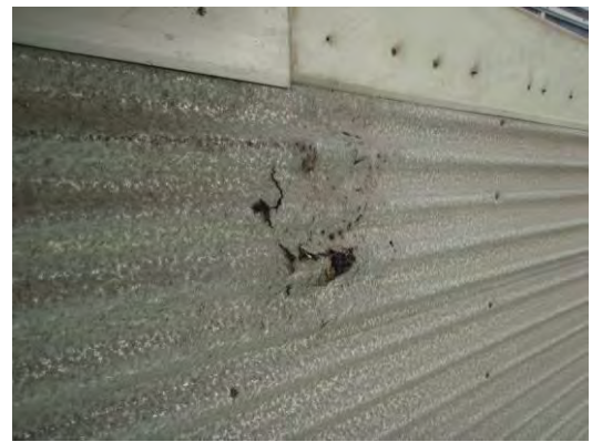
Figure 48 Grandstand Roof Corrosion
