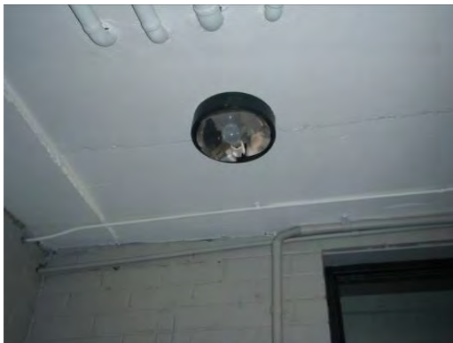
Figure 18 Light Fitting Missing Diffuser
