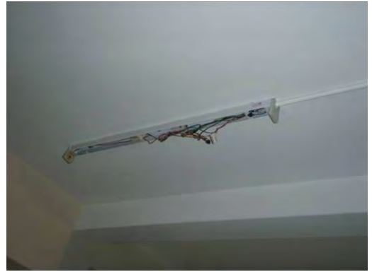
Figure 17 Light Fitting Cover Missing
