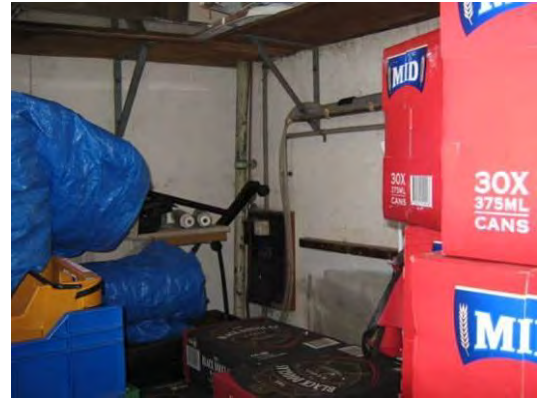
Figure 37 Drink Store Electrical Switchboard
