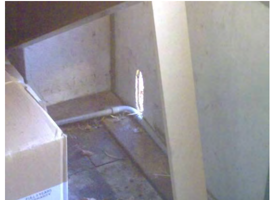
Figure 46 Hole in Wall Below Fire Stair from Function Room
