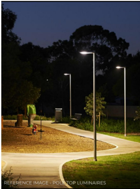
Figure 6: Reference Image - Pole mounted Luminaires
