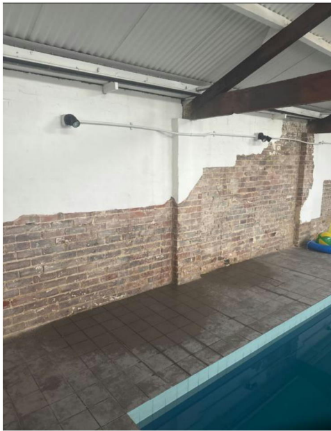
Image – Existing Parapet wall and water damage
