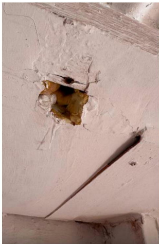
Image– Existing boxed gutter Broken gutter
