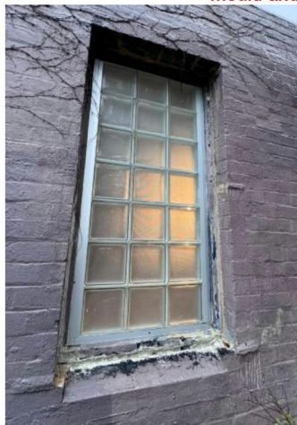
Image– Existing glass blocks to façade shows evidence of water damage boxed
