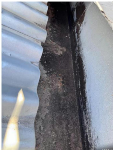
Image– Existing boxed gutter
