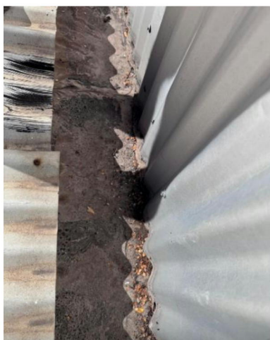
Image– Existing boxed gutter
