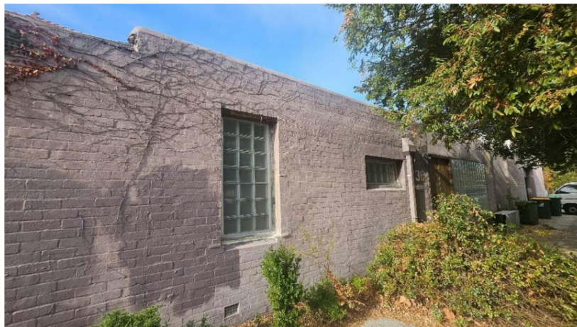
Image – Existing Façade – Washington St – water damage evident on existing wall
