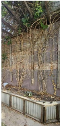
Image – Existing Landscaping to be removed, and new landscaping to be provided to reduce further destruction of the structure
