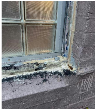
Image – Existing opening damaged by water
