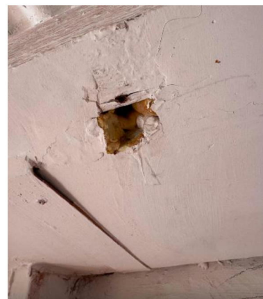
Image – Existing broken boxed gutter
