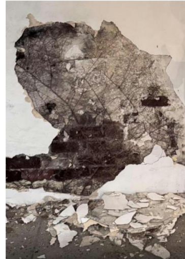
Image – Existing plaster cracking water and roots damage
