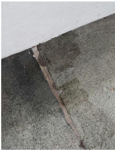
Image – Rising damp existing slab
