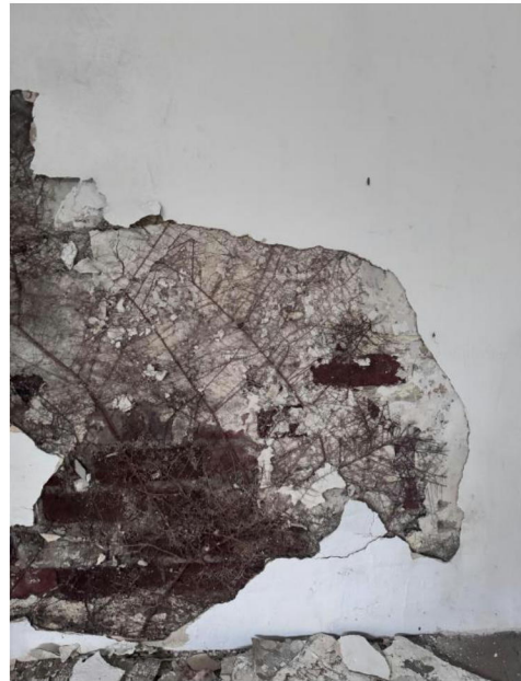
Image – view of front façade damage, internal, water and mould and plant root Existing Façade – Washington Street
