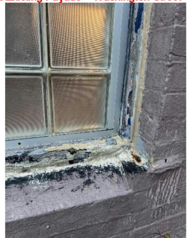
Image– shows extent of damage
