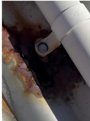
Image – Existing roof corroded and broken
