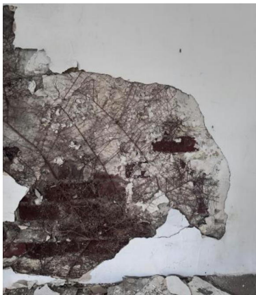
Image – Plaster damage and mould to inside face of façade parapet wall
