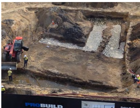
Plate 11. Exposed section of Barrack Street Jetty and River Wall from Perth Bell Tower
