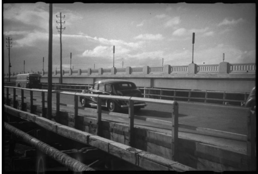
Figure 28. 1950s Causeway Bridge II still in use while Causeway Bridge III is under construction, showing broken railing (slwa_b6058475_1)
