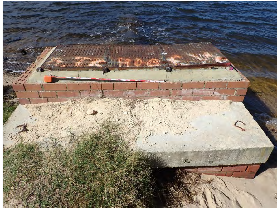
Plate 8. View east of modern brick and concrete structure with drain pipe extending into the Swan River
